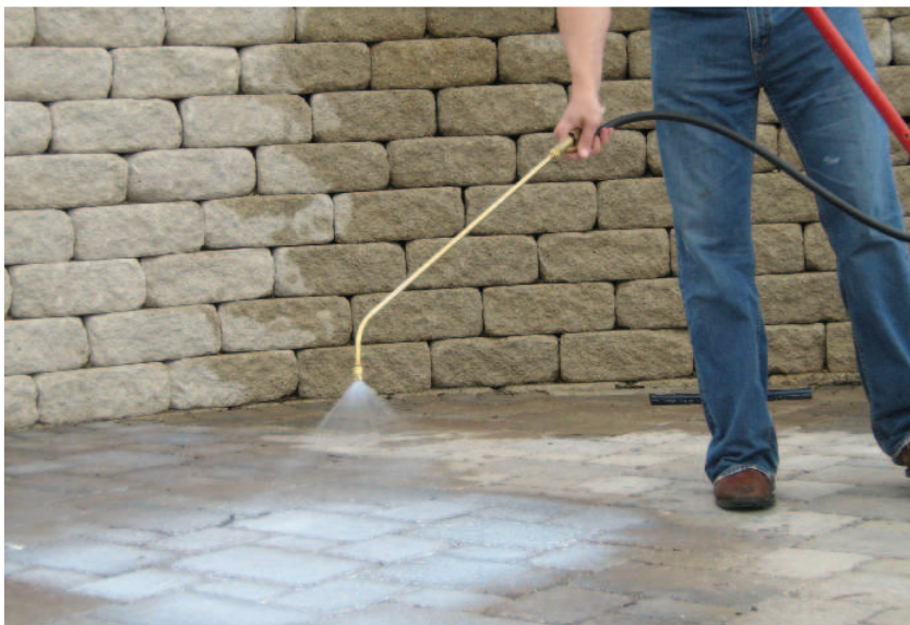
Spraying sealers can help achieve a consistent coat and can be faster than rolling the sealer onto the concrete.
